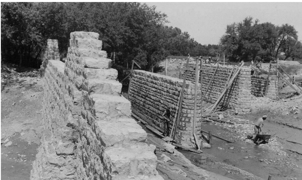
Figure 29. Use of stone masonry on THD project in Erath County, late 1930s. (Source: Texas Department of Transportation Photo Library)
