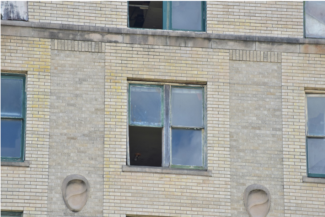
Photo 16. East elevation, detail of masonry at eighth floor, columns and cartouches, view west, 2017.
