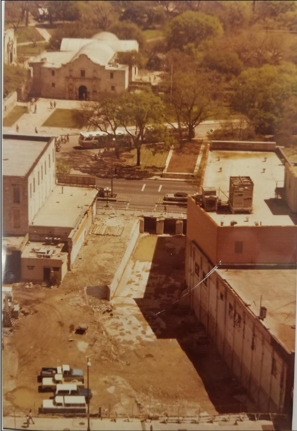
Figure 16. Site of CAR's 1979 excavations during construction of Lower Paseo, facing east. (Photo on file at CAR)
