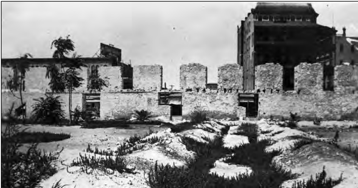
Figure 12. View of Convento/Long Barrack after the demolition of east exterior wall and before demo of the second story in 1913. (General Photograph Collection, UTSA Special Collections)
