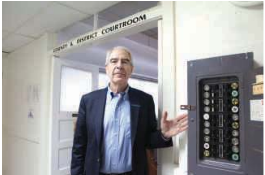
Judge Byron Theodosis with the obsolete plug fuse electrical panel outside San Saba County's County and District Courtroom. Workers must flip switches on this panel to control the lights in the courtroom. (Photo by Liz Carmack.)
