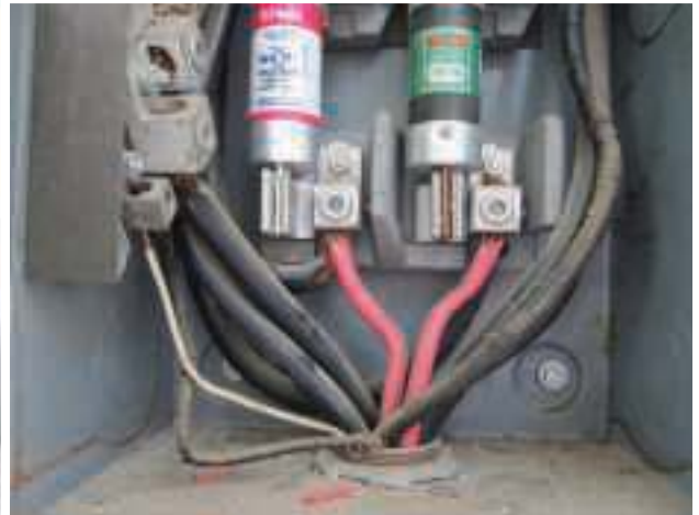
Electrical wiring, switches and panels shown in the courthouse's original service entrance that are considered a safety and fire hazard because of exposed live parts, cloth covered feeder conductors with deteriorating insulation, unlabeled equipment and other issues. (Photos courtesy Architexas.)
