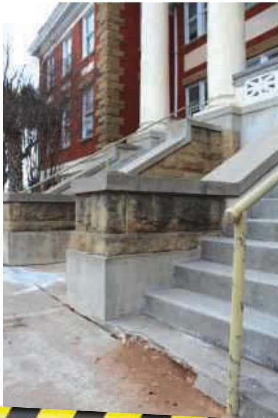
Crumbling and cracked concrete on the building's exterior stairs and sidewalks are on the list of immediate repairs needed to improve safety at the San Saba County Courthouse. (Photo by Liz Carmack.)
