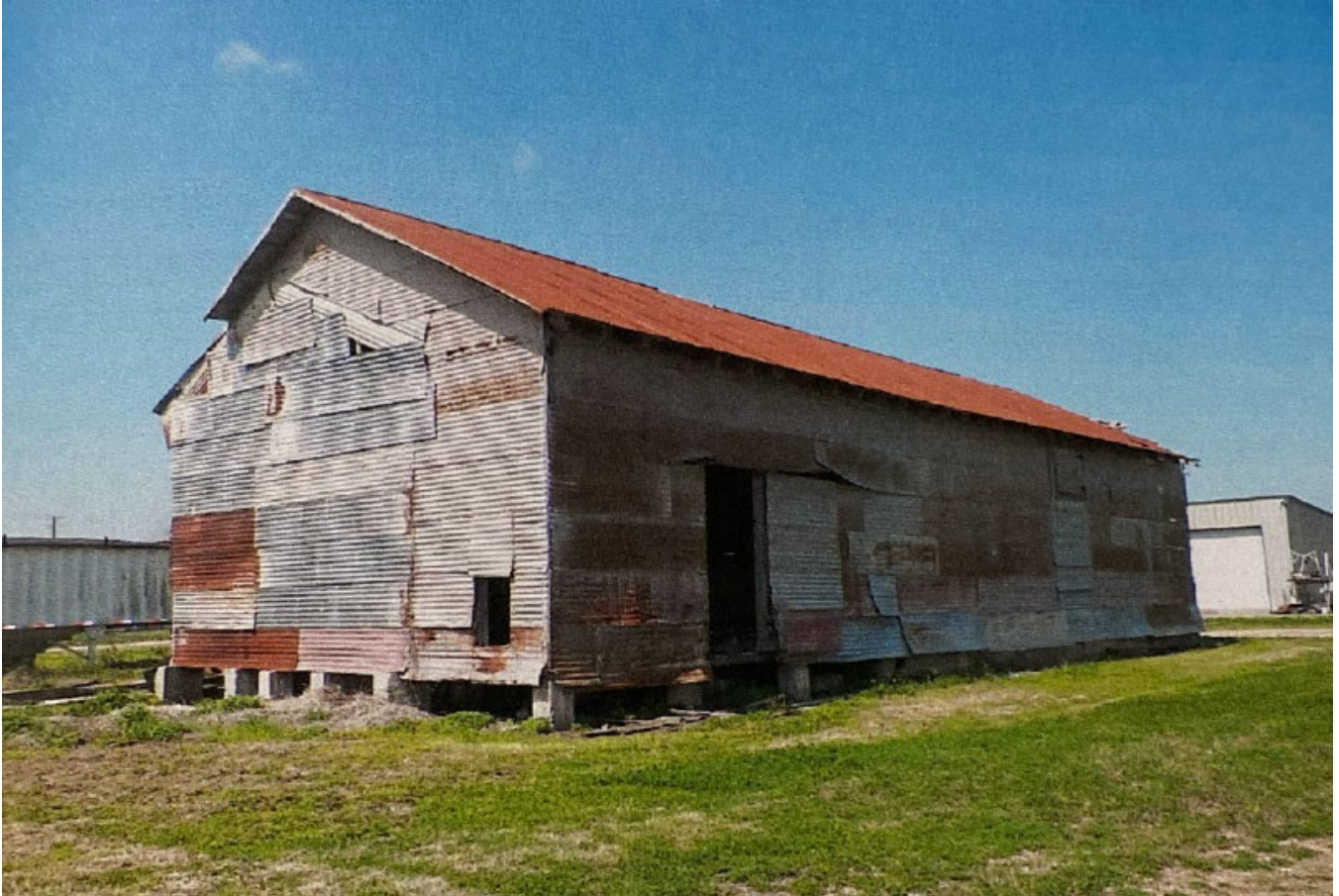
Figure 39. This image shows the current condition of the Farmers Gin building that operated between 1944 and 1951 at the intersection of State Highway 87 and Gin Road (Spiller 2014).
