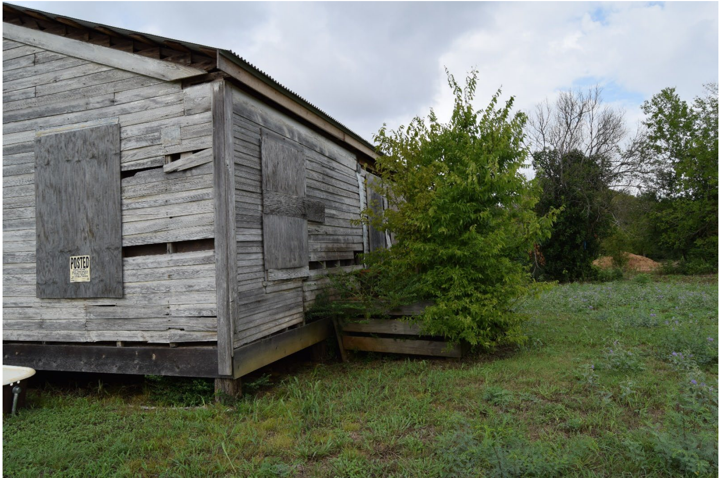
Photograph 25. Beveled-shoulder cistern at north side of house, obscured by foliage. Camera facing west.
