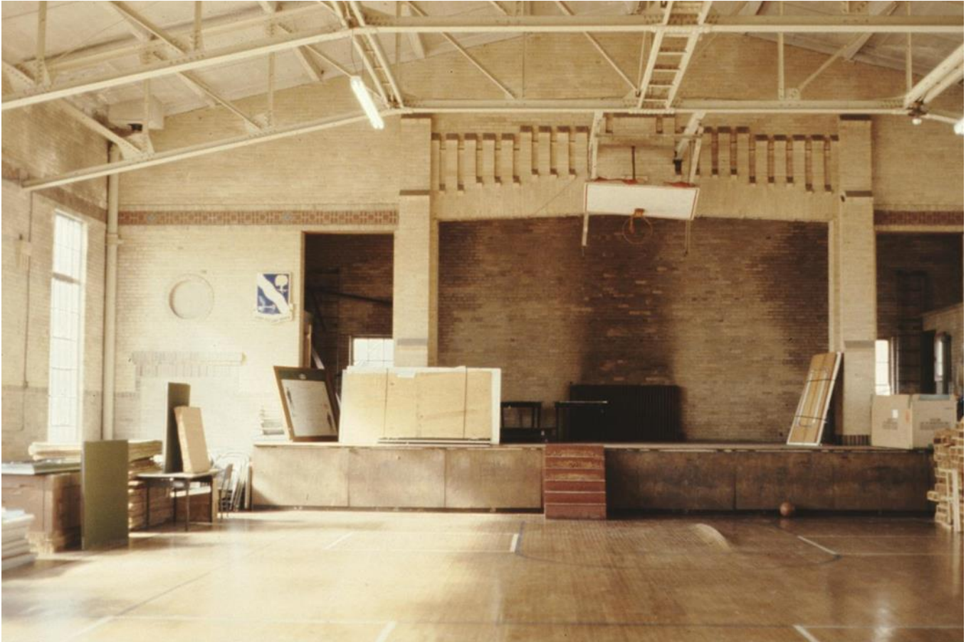
Figure 6. The stage in the drill before renovation, unknown date. Source: Texas Historical Commission. [Light Guard Armory], photograph, unknown date; ( https://texashistory.unt.edu/ark:/67531/metaph949447/ : accessed February 9, 2023), University of North Texas Libraries, The Portal to Texas History, https://texashistory.unt.edu ; crediting Texas Historical Commission.
