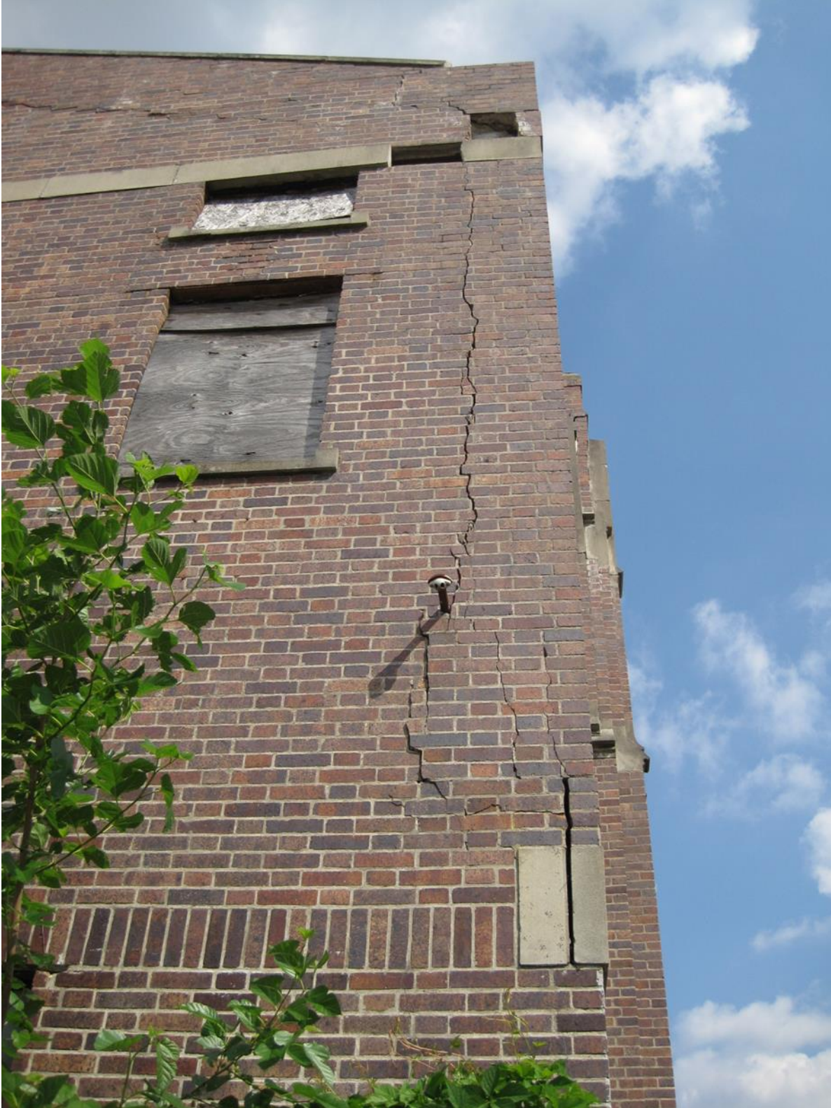
Figure 10. Brick separating at the rear (northwest) façade in 2010. Source: Texas Historical Commission.
