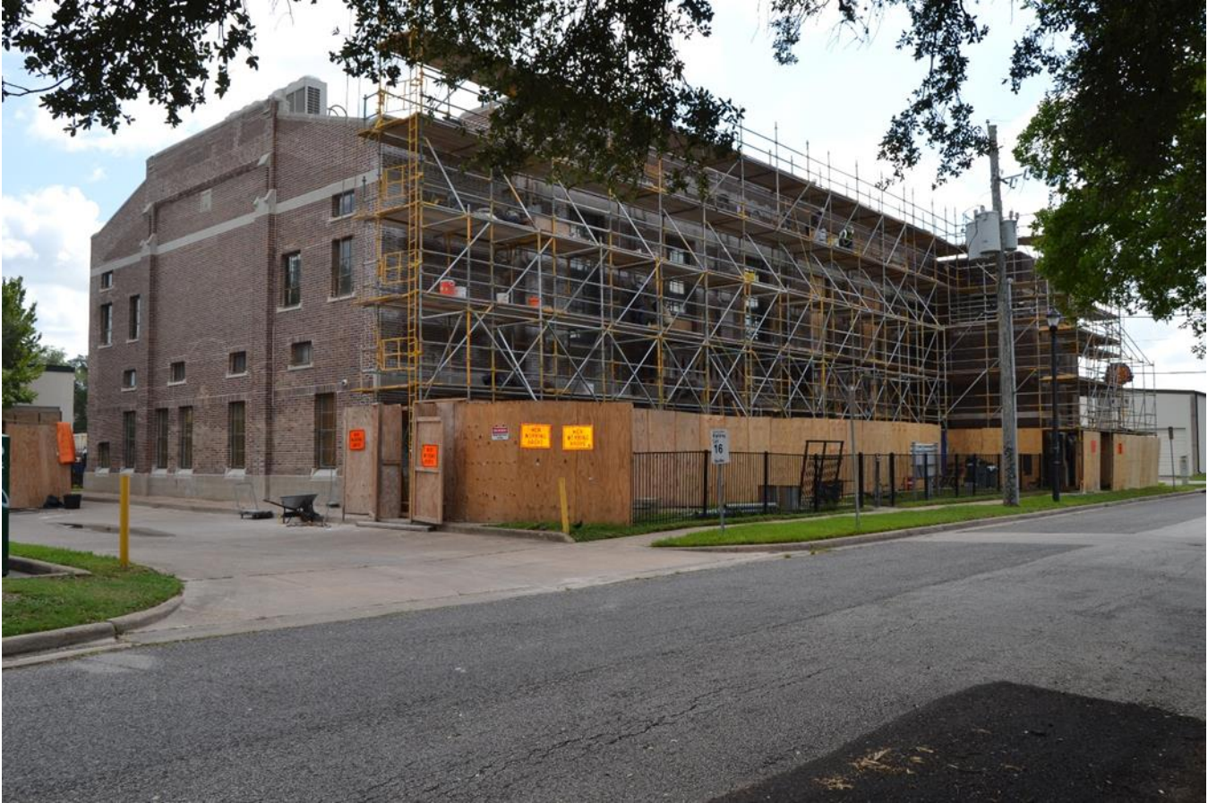
Photo 10. Oblique of the side southwest and rear northwest façades. Camera facing northeast.
