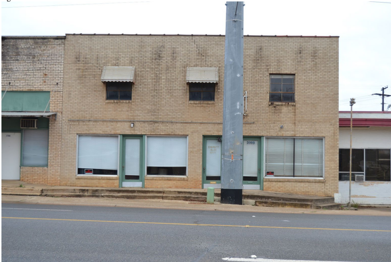
Photo 14. Camera facing north showing Resource 7 at 3705-07 West Marshall Avenue. Resource 8 is pictured to the right.
