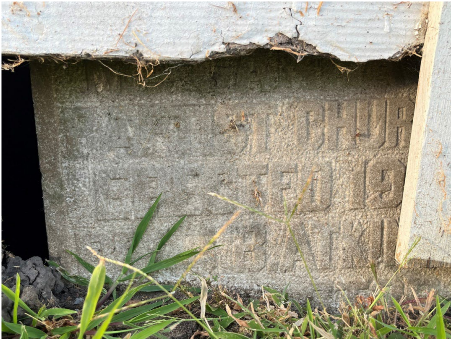
Photo 6: Original cornerstone beneath siding on the north elevation. "Mt. Canaan Baptist Church, Erected 1910, Rev. M.B. Atkins"
