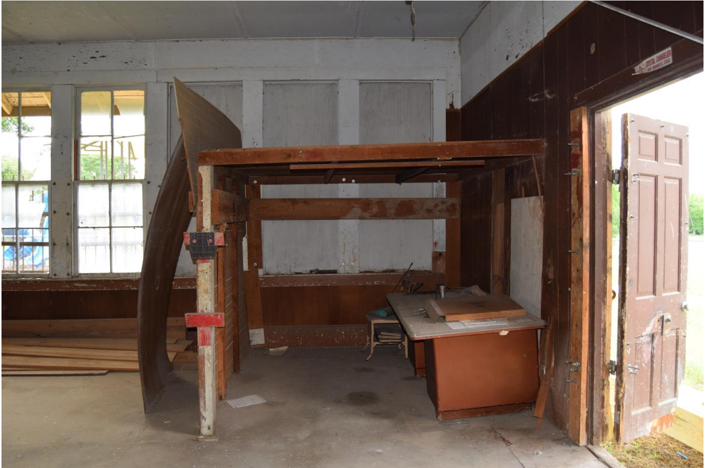
Photograph 12. Partition walls at south end of southeast interior wall, view facing southeast.
