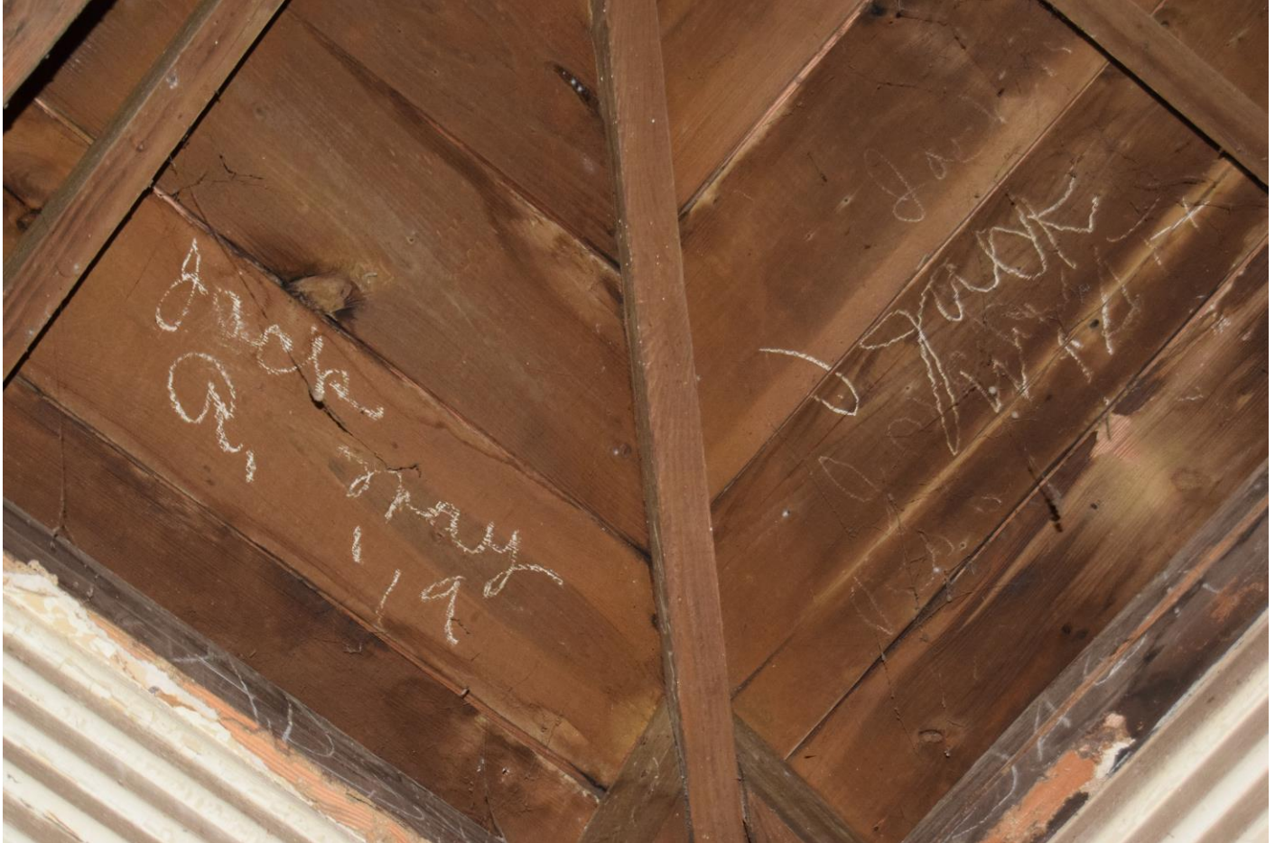
Photograph 17. Roof structure on interior of closet at south end of northwest wall, view facing southwest.
