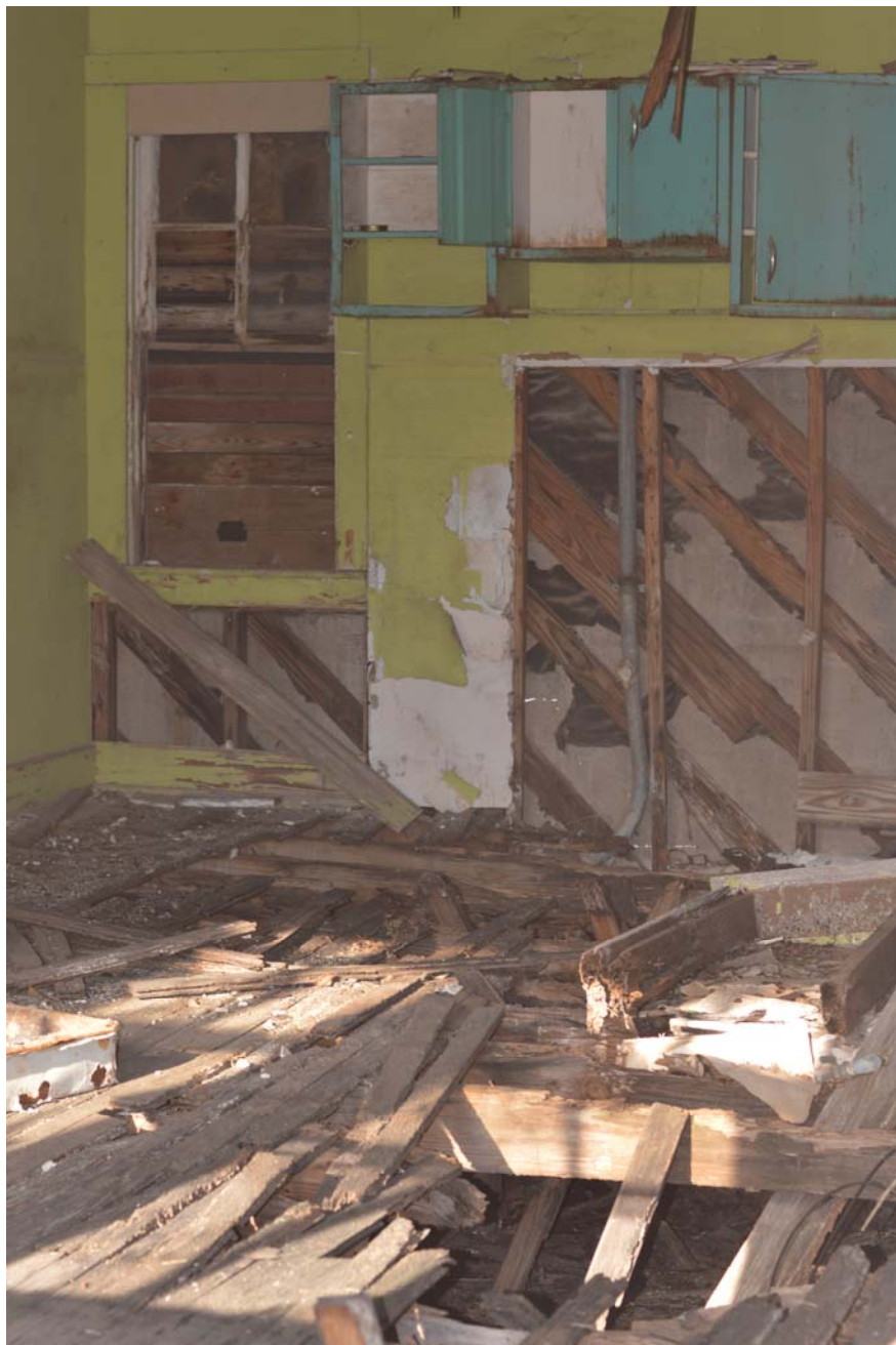
Photo 14 Typical condition in rental units, with deteriorated flooring
