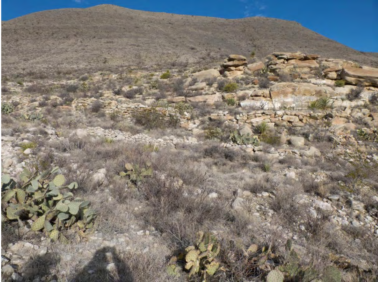
Photograph 12: Overview of Eastern Slope located below Guadalupe Pass showing Road Segments 10 (2CC) and 13 (2FF) with stone retaining walls and fill.
