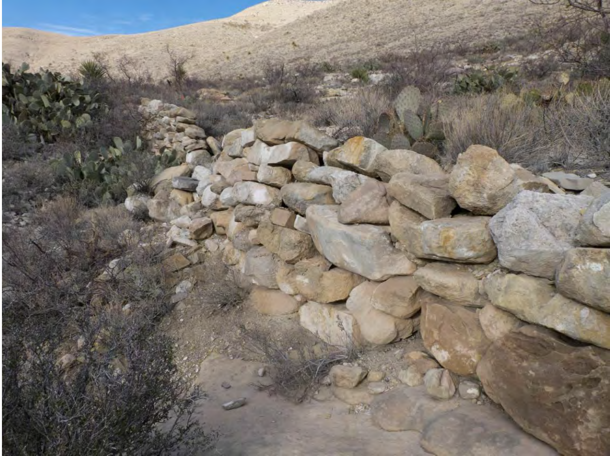
Photograph 9: Detailed view of Road Segment 10 (2CC) and its stone retaining wall and fill (2R)
