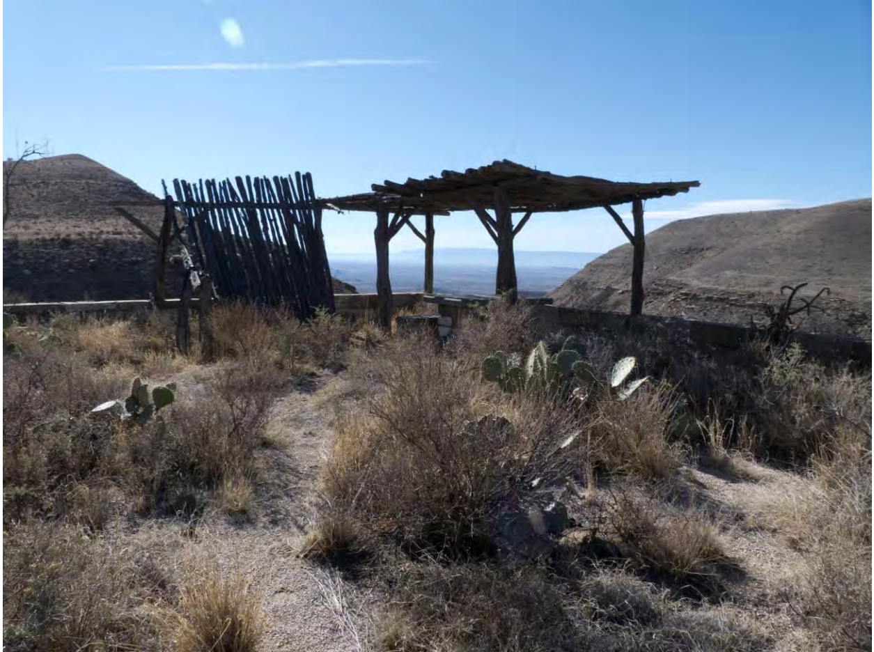
Photograph 5: Polancio Park (Signal Peak Roadside Park) Ramada 2 Ruins (2A)
