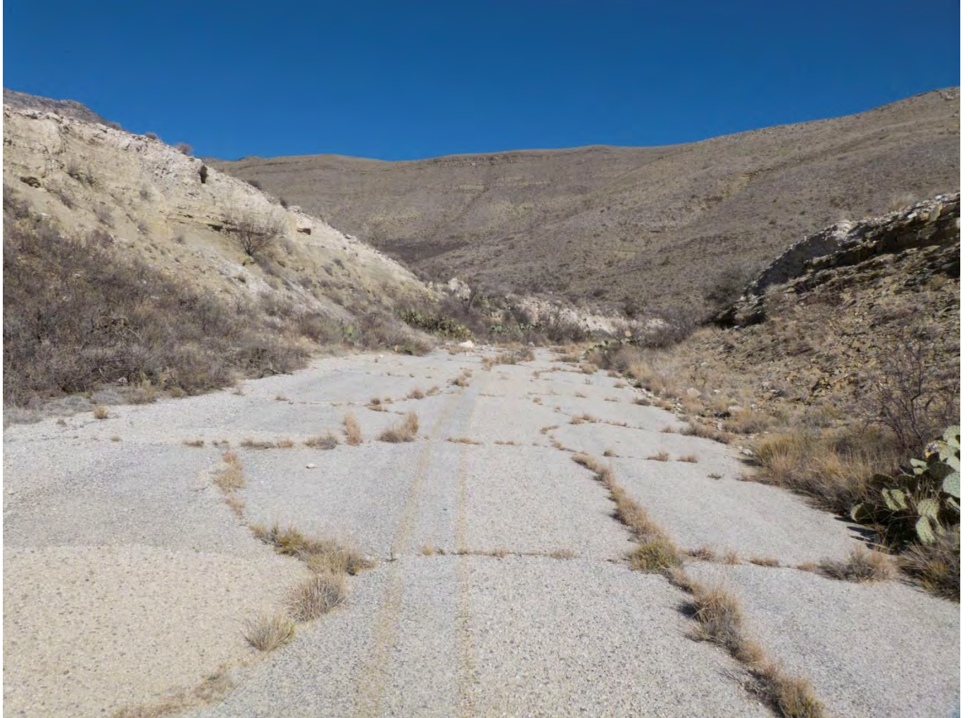
Photograph 22: Overview of Road Trace 1/2U - 1937 alignment of Highway 62 showing superelevation and pavement.
