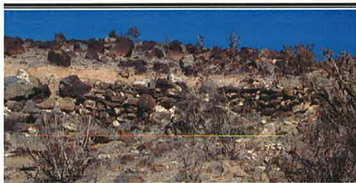
Retaining wall on La Bajada allowing motorists on U.S. 66 to gain a slightly better hold on the road. Photo: Michael Cassity, 2004.
