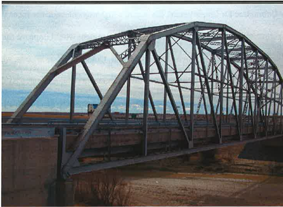
Rio Puerco Bridge, west of Albuquerque, completed in 1933. An example of the property type Bridges, this is a splendid Parker Camelback Through-Truss bridge. Photo: Michael Cassity, 2004.
