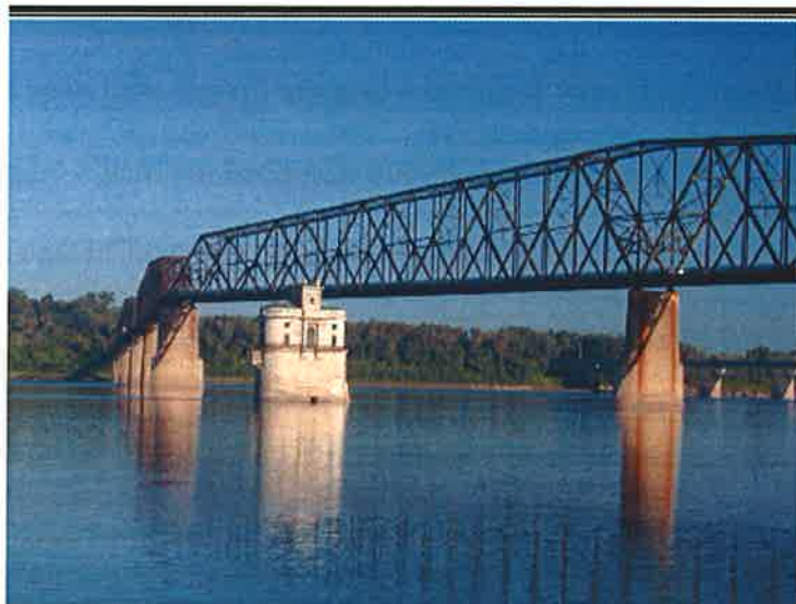
Chain of Rocks Bridge (1929) showing bend in bridge. Photo: Michael Cassity, 2004.
