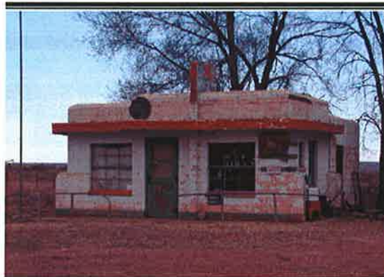
Abandoned café, Glenrio, Texas (1930). Suffering from the deterioration common to buildings no longer in active use, this café was at one time a gasoline station and also a trading post for curios, a common occurrence reflecting changing times and traffic on Route 66. Photo: Michael Cassity, 2004.
