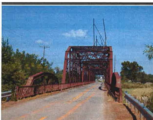
Lake Overholser Bridge, Oklahoma City (1924-1925) replaced a ferry across the North Canadian River. The bridge is a combination of camelback Warren pony trusses on each end and four Parker through-trusses between. Photo: Michael Cassity, 2003.
